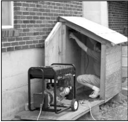
Gill Jeffer really getting "into his work" on the emergency generator shed.
